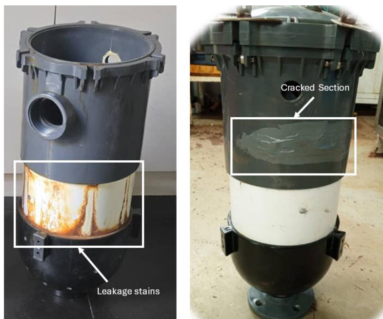
Figure 1: Leakage stains and cracks present on the failed filter bag housing
